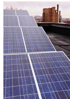
Figure 3. PV array on Dana Building 25
